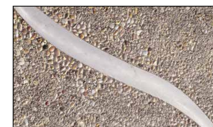
Steel bands embedded in the concrete mark the 'guitar strings' across the plaza and would incorporate an in-ground lighting system for a dramatic night-time effect
